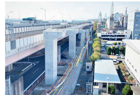
FY2020 Route 247 Nishi Chita Doro Tokai JCT/H Lamp Bridge Lower Part Project Tokai City, Aichi Pref. Client: Chubu Regional Bureau, Ministry of Land, Infrastructure and Transport
